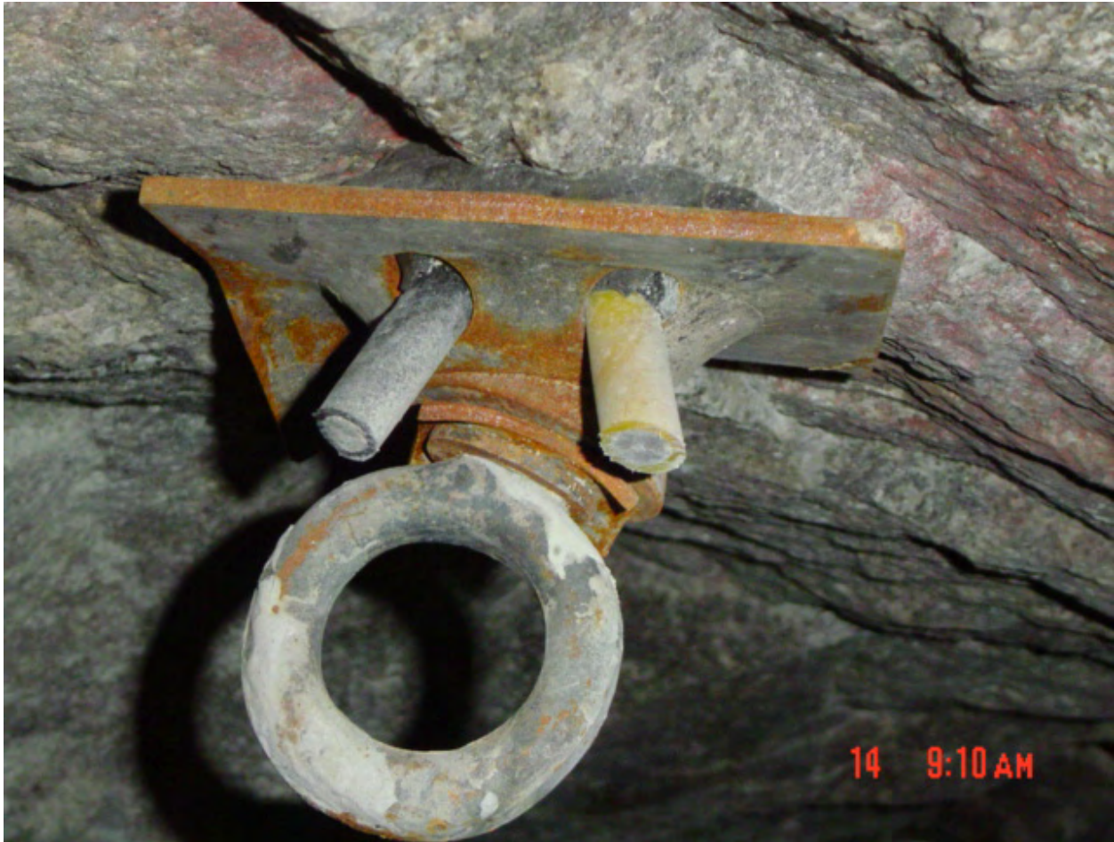
AN EXCELLENT EXAMPLE OF A GOOD INSTALLATION
